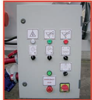
MAIN CONTROL SYSTEM
