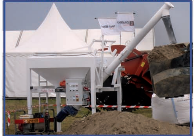
EASILY CONNECTS TO GENERATOR ON SITE.
